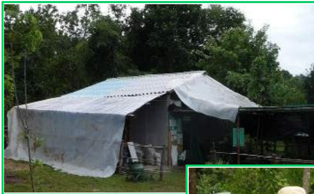
Above: the nursery in Kaeng Plakod village being re-roofed with plastic and concrete tiles.
